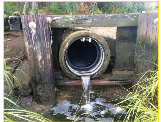
A 48" ProFlex 790 installed and operational, ensuring backflow protection against wave action and rising water
