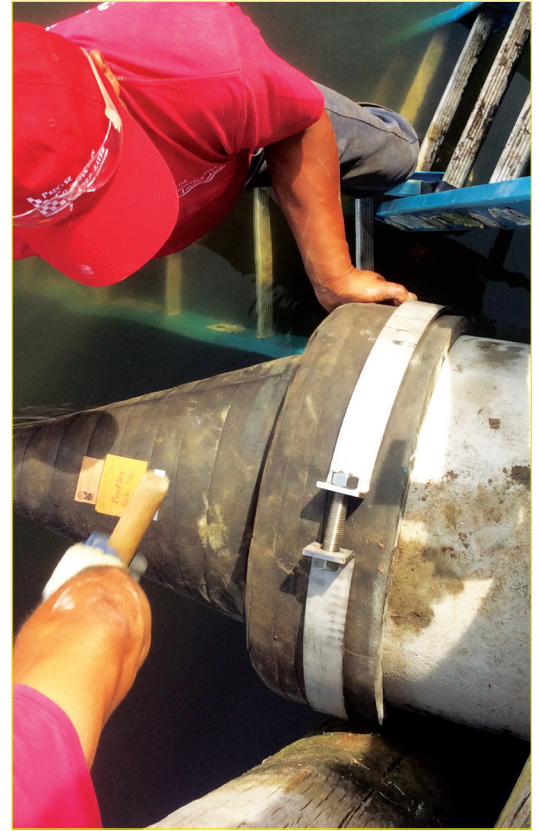
A perfect install, SS clamps being fitted to ensure secure attachment to the pipe
