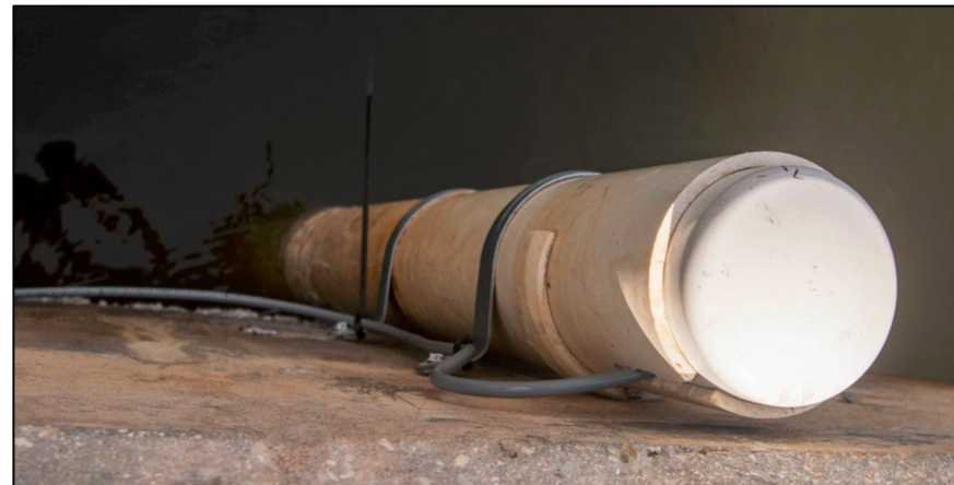
Level sensor housed in a PCV cylinder fixed to structure.
